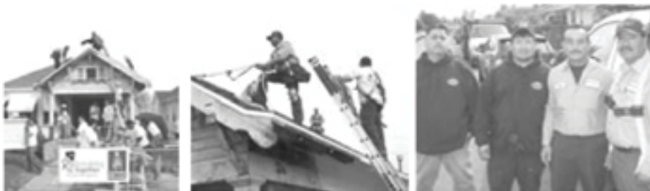
Expert roofers from URCA contractor companies—Best Contracting Services, Eberhard, Chapman Coast Roof Co., Alcal Arcade Contracting, Anning Johnson, and Empire Contracting participated in the Central Los Angeles "Rebuilding Together" project.
